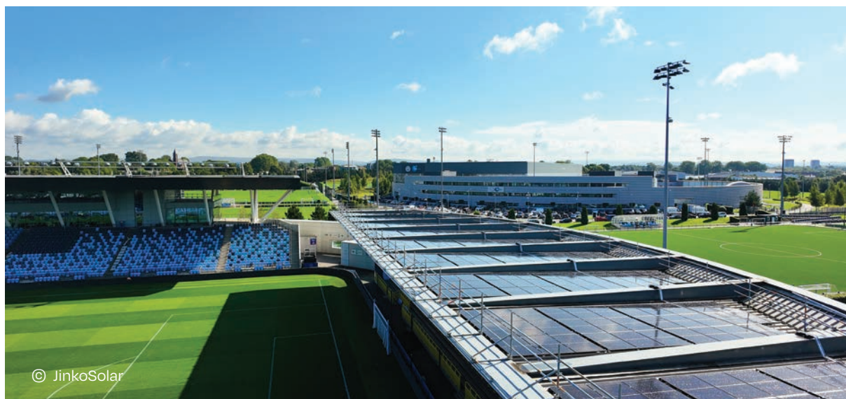
PV system on Joie Stadium, Manchester, UK
