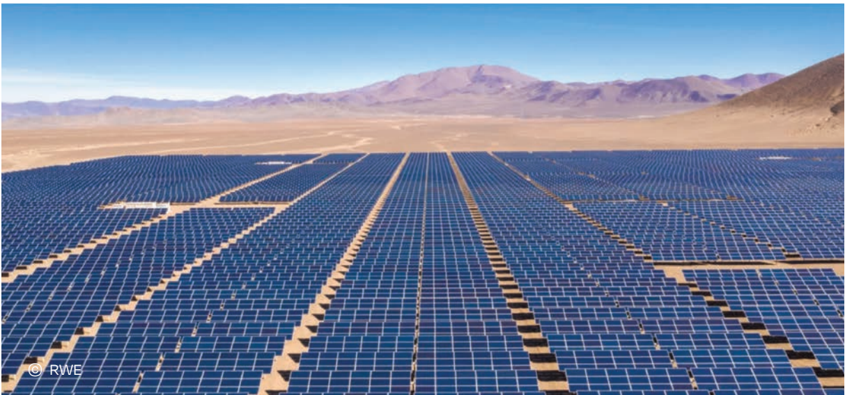
269 MW coupled with 1.1 GWh BESS Oasis de Atacama solar park, Chile
