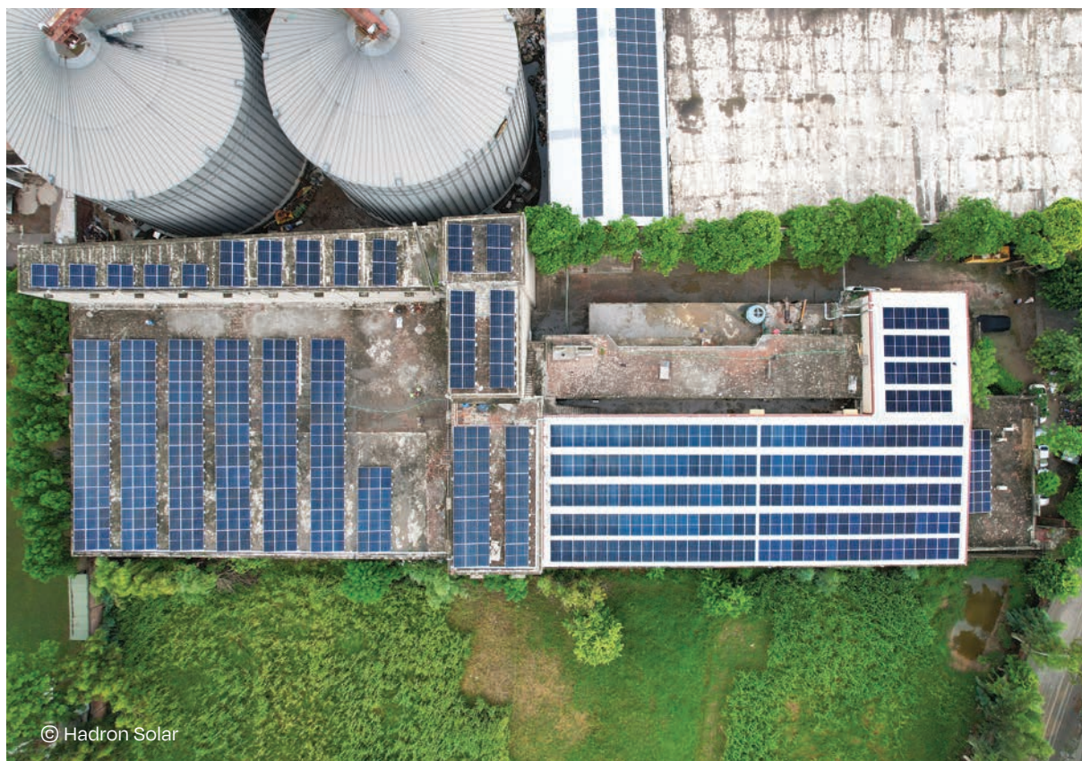
286 kW Qamar Fabrics solar plant, textile factory in Lahore, Pakistan
