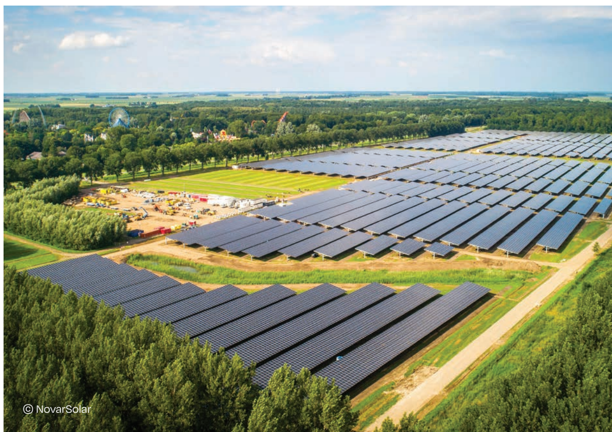
37.7 MW solar PV carport, Biddinghuizen, the Netherlands
