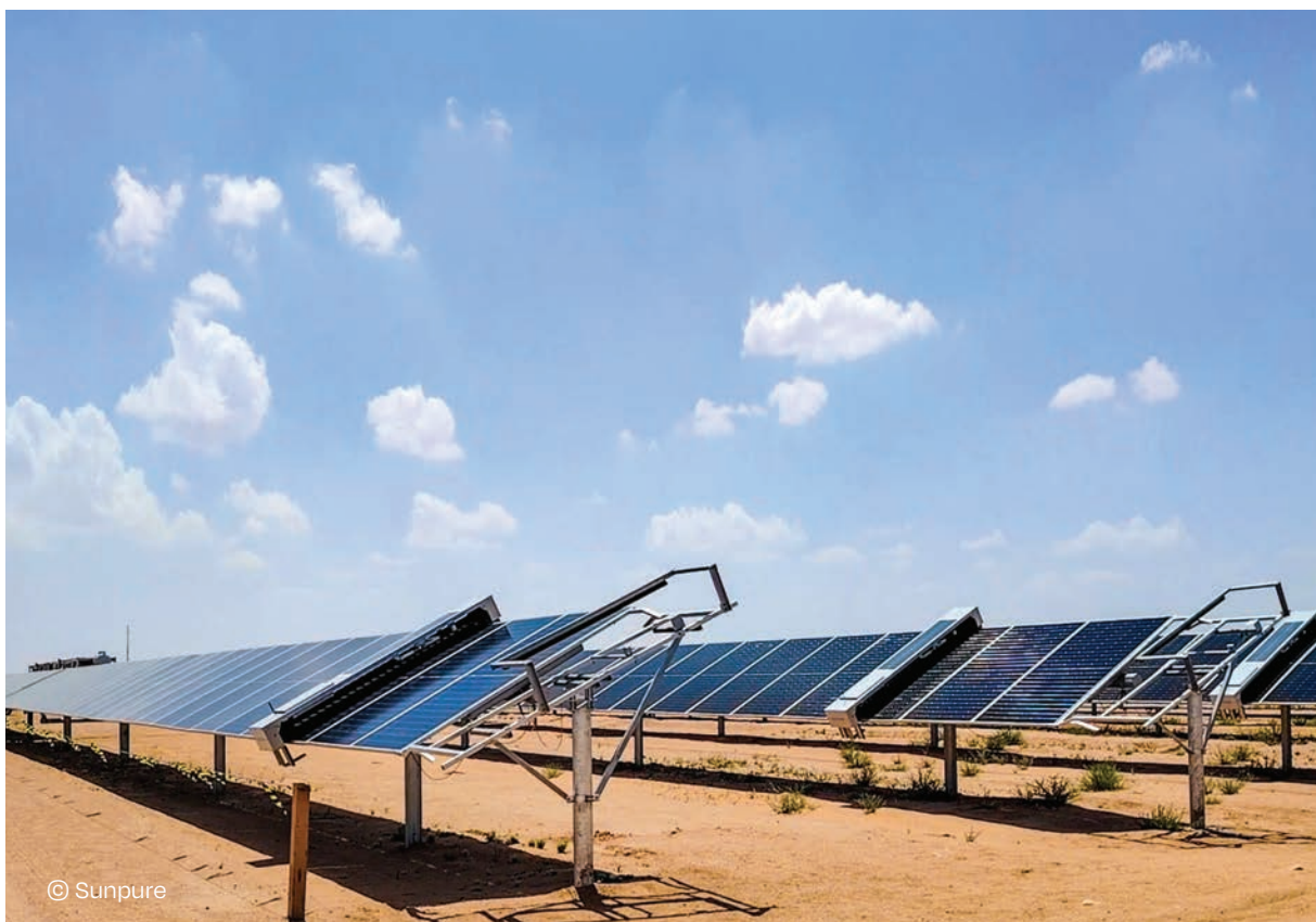
PV cleaning robots, Saudi Arabia
