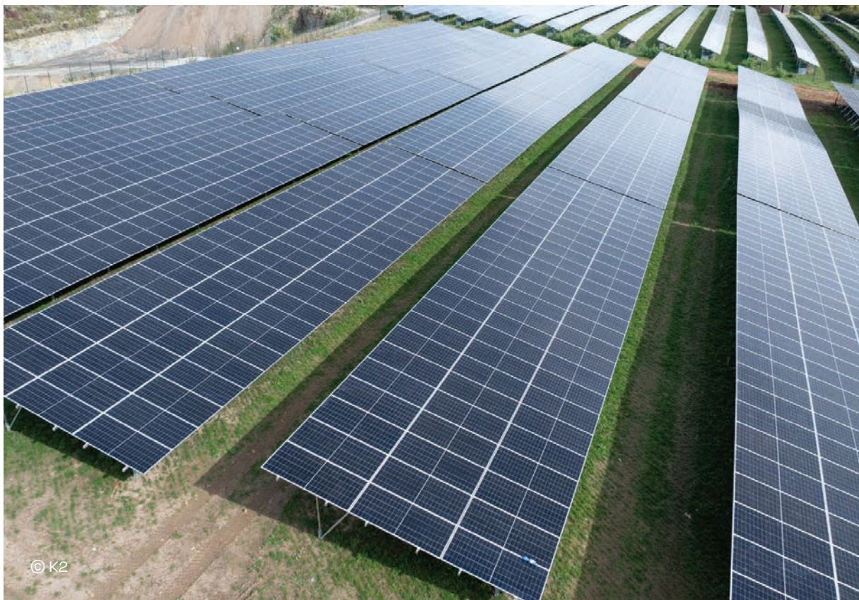
1.5 MW, Illingen, Germany
