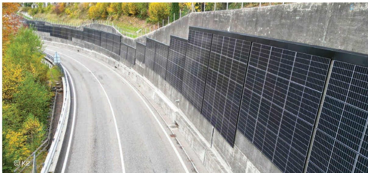
325 kW, Ausserrhoden, Germany
