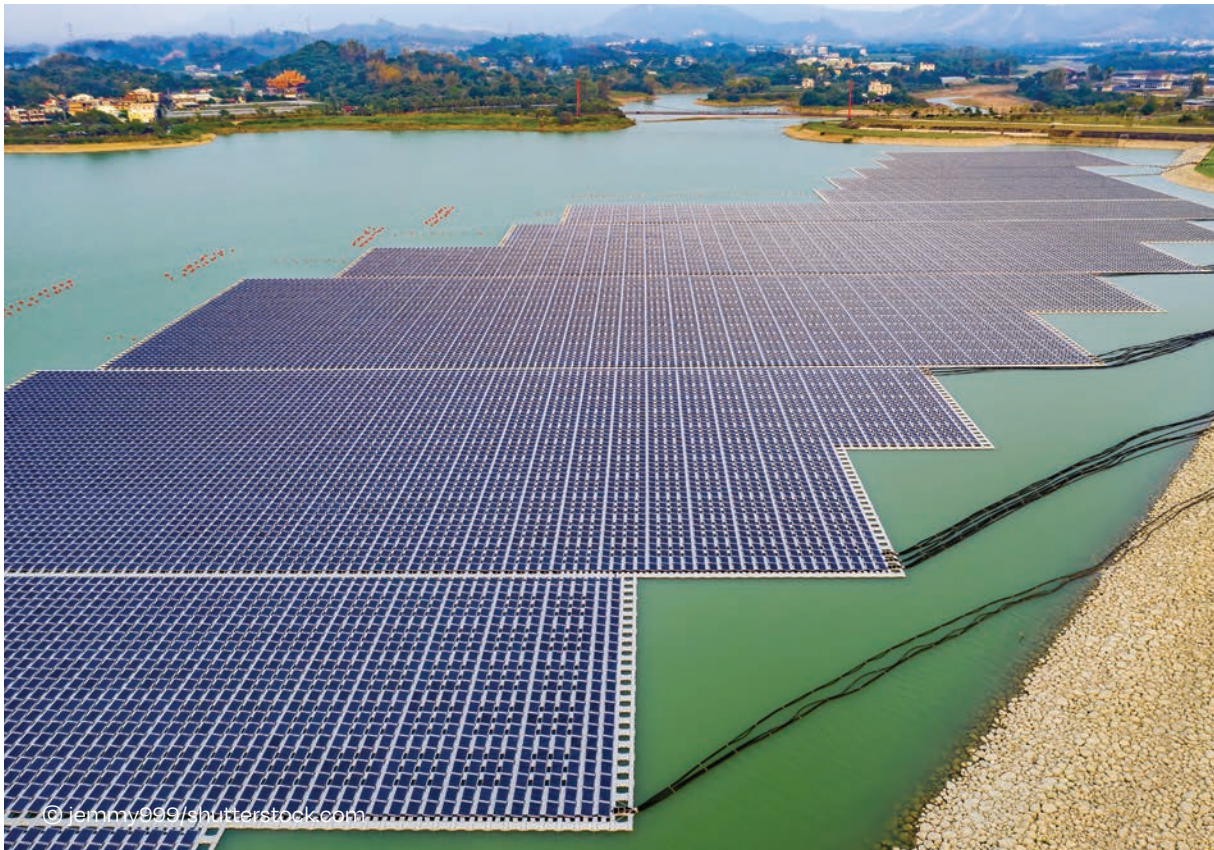
10.02 MW Agongdian solar PV park, Kaohsiung Reservoir, Taiwan.
