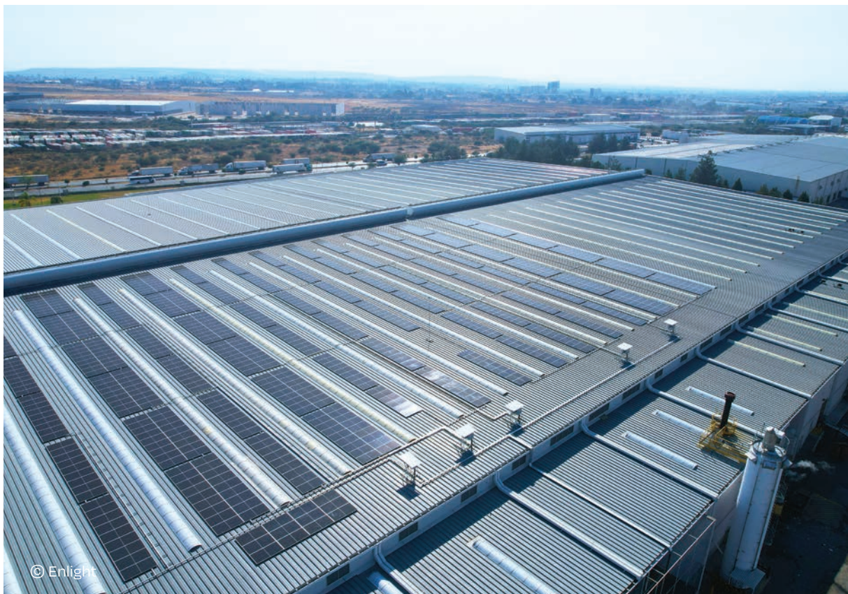
550 kW solar plant for paper and carboard industry, Guanajuato, Mexico
