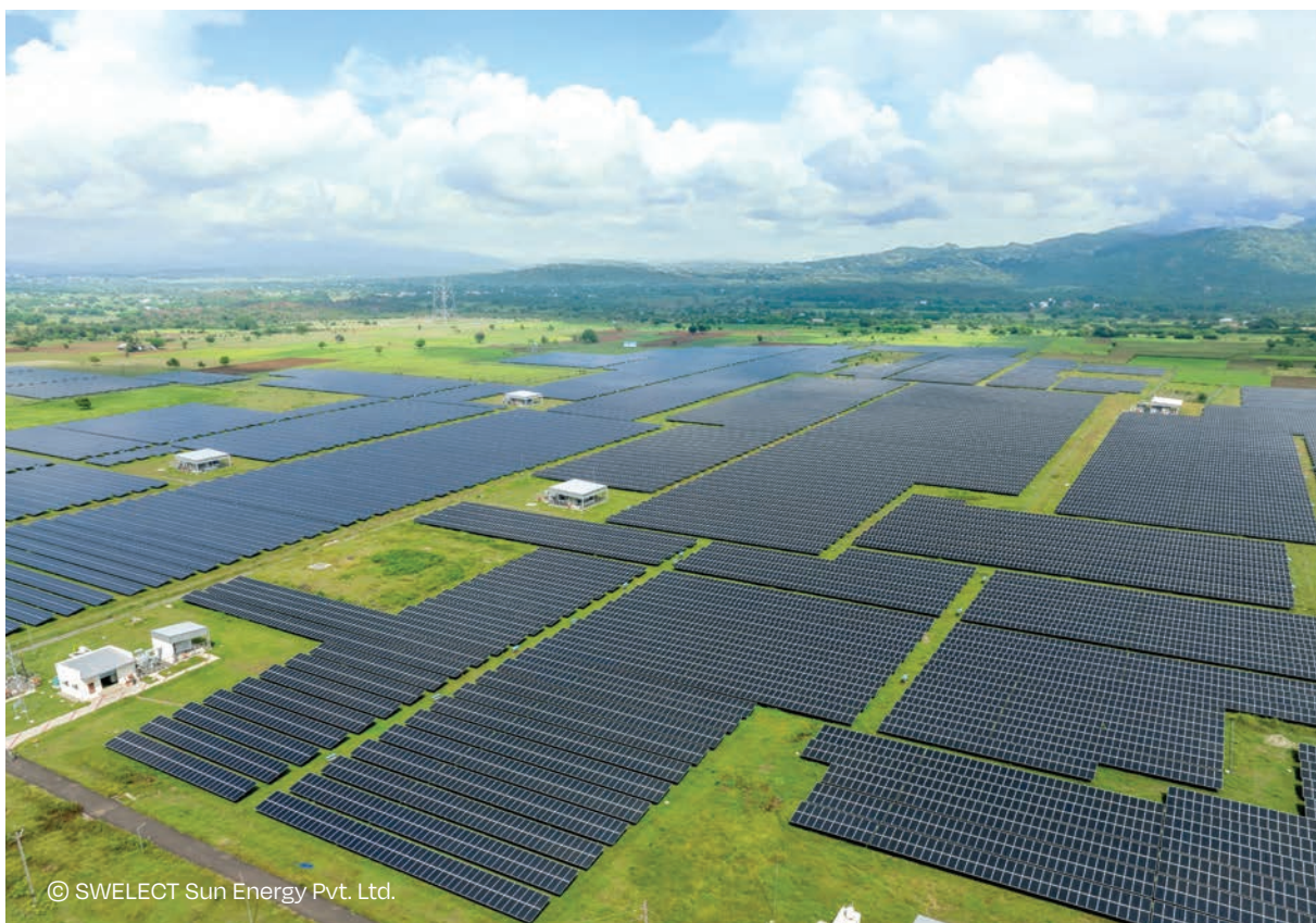
6 MW solar project, Vengaimandalam, Trichy, Tamil Nadu, India
